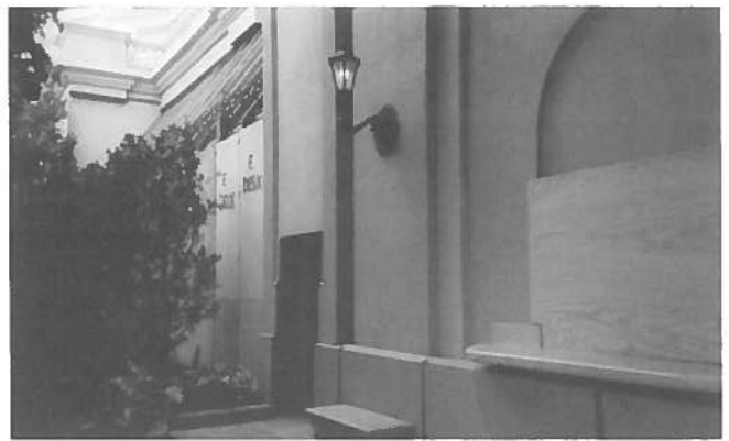
Front windows of Beau Rivage boarded up
