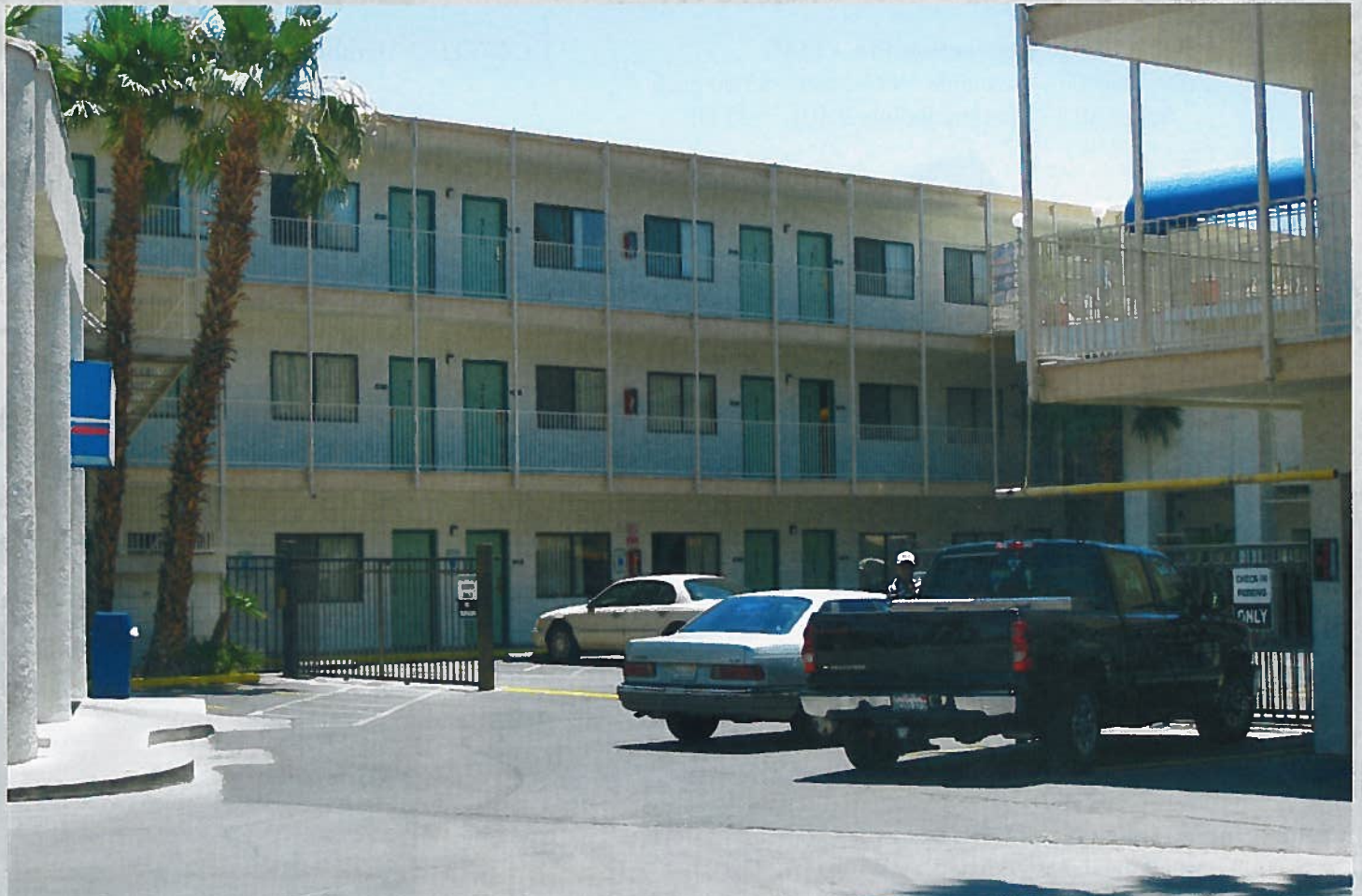
A close up view of the hotel rooms that were effect by the bomb blast in 1967. Photos on this page provided by Marc Shapiro.
